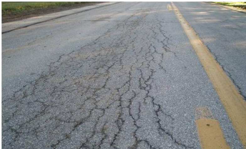
Figure 4. Load-associated fatigue cracking (Road Science 2015)
