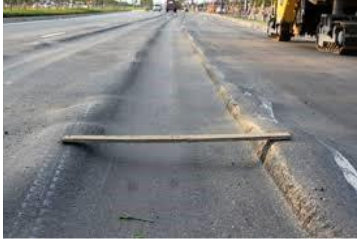
Figure 3. High temperature pavement deformation (rutting) (BMT 2013)
