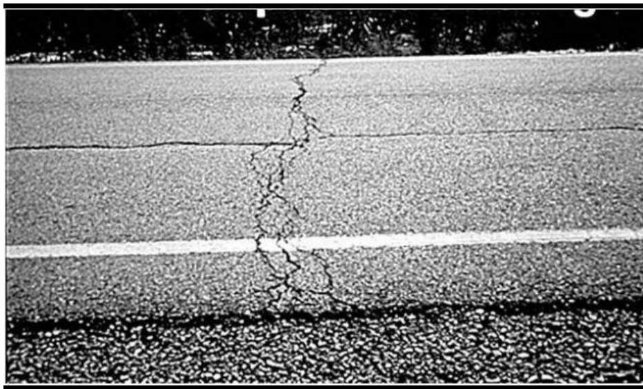
Figure 5. Low-temperature thermal cracking (Road Science 2015)
